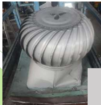
TURBINE VENTILATION SYSTEM
